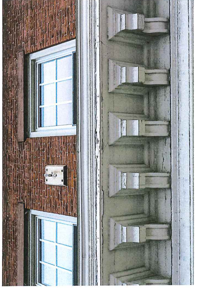
West (Front) Entrance Cornice Water Damage
