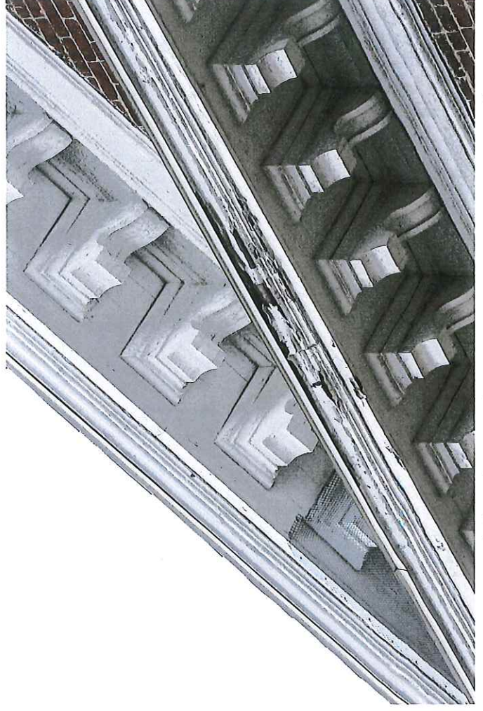
South (Academy St.) Cornice Water Damage - Detail
