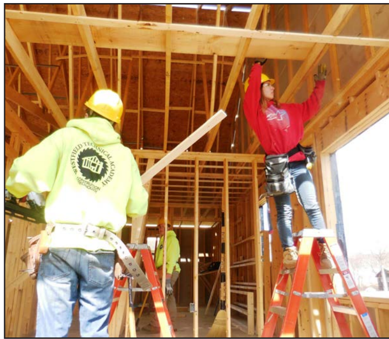
Westfield Technical Academy students working on the interior are, A. J. Onofrey and Sara Whalen.
