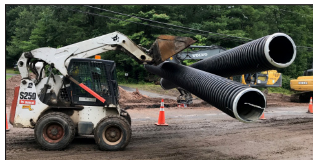
Pereira Construction is seen delivering the piping for the drainage on Congamond Road on Monday morning. (Photo by Greg Fitzpatrick)
