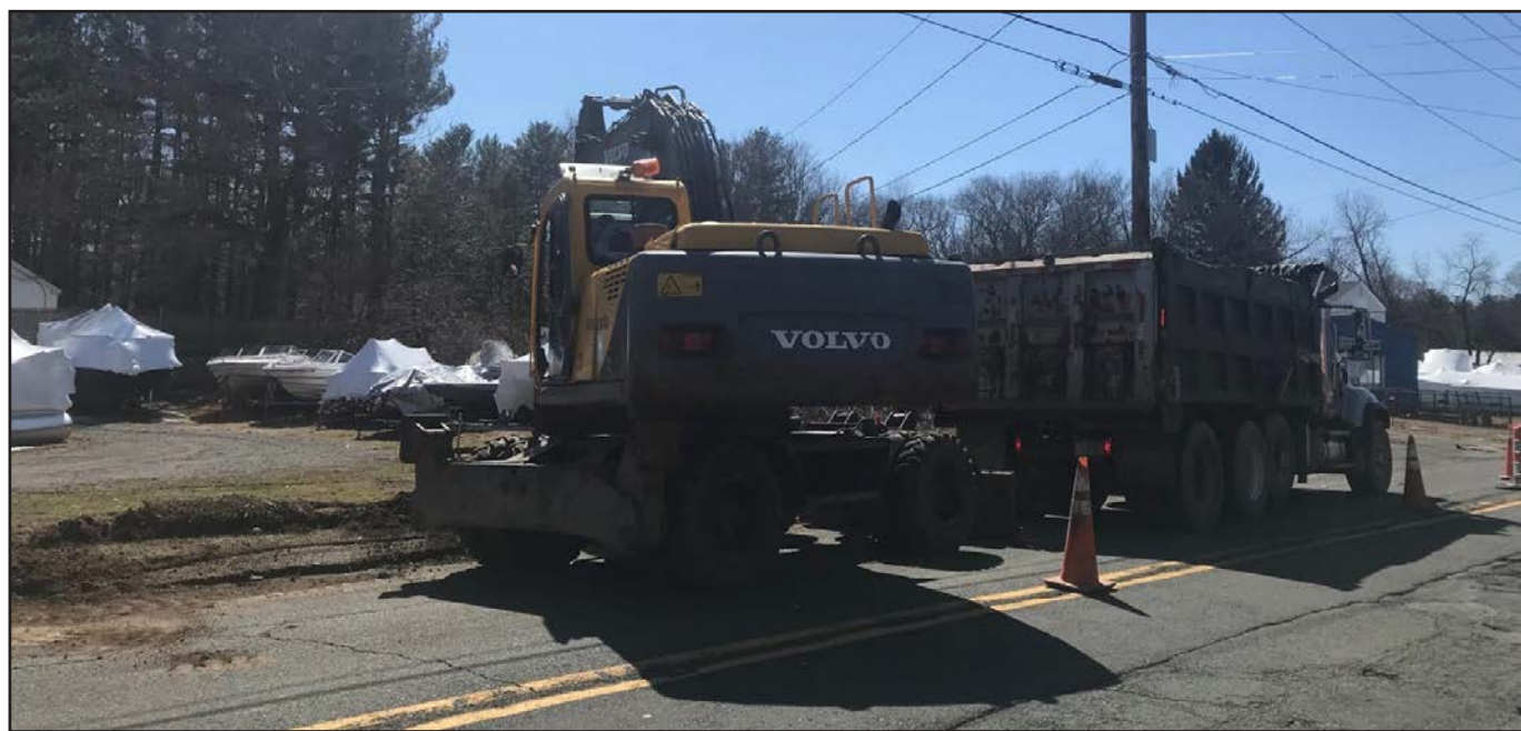
Workers from Pereira Construction are seen widening Congamond Road on Monday afternoon. (Photo by Greg Fitzpatrick)
