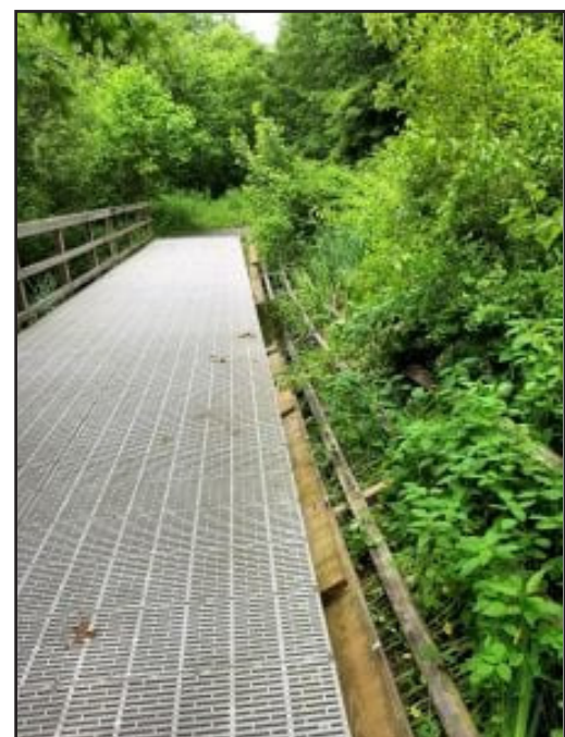
The railing on this bridge at Grandmother's Garden was vandalized last week. (Photo by Richard Holcomb)
