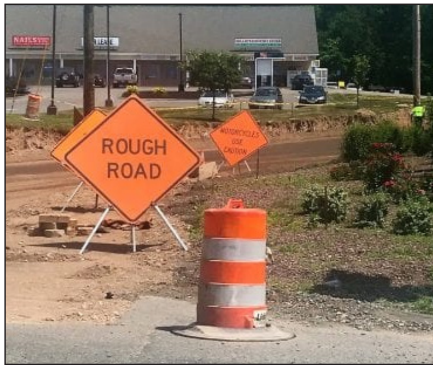
Road improvements on Congamond Road in Southwick are part of a transportation bill approved July 16 in the Senate. (THE WESTFIELD NEWS PHOTO)
